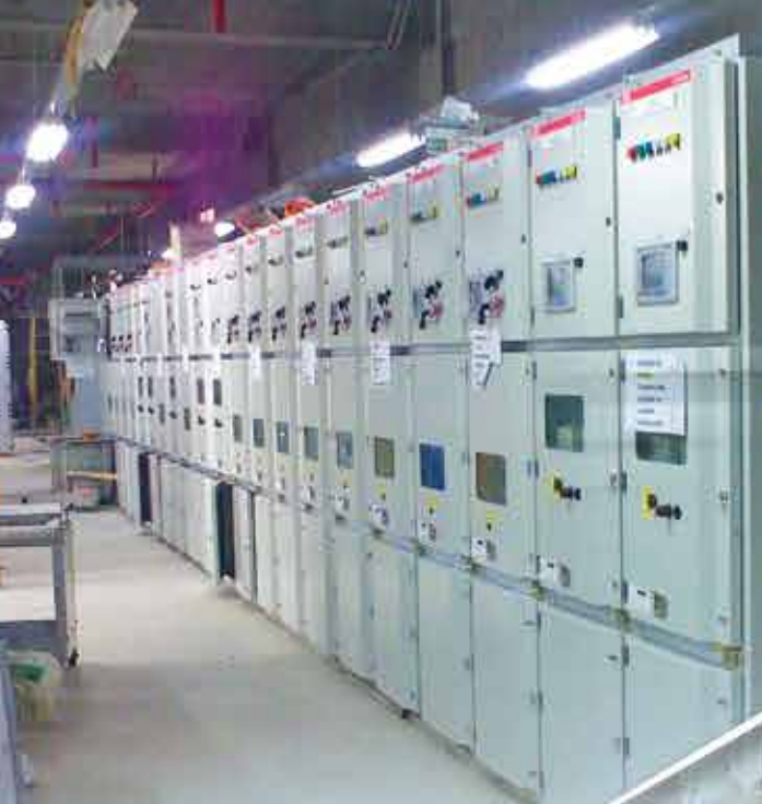
HV & LV OF DISTRIBUTION PANEL IN SUBSTATION
